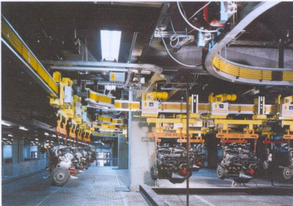
Back-up line installation of an electrically driven trolley conveyor for the transport of motors.
