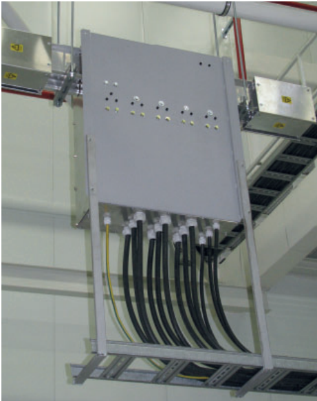
Centre feed made to accommodate multiple cables.
