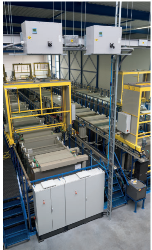
Power Xpert® XP Tap-off units feeding the switchboards with process control equipment.
