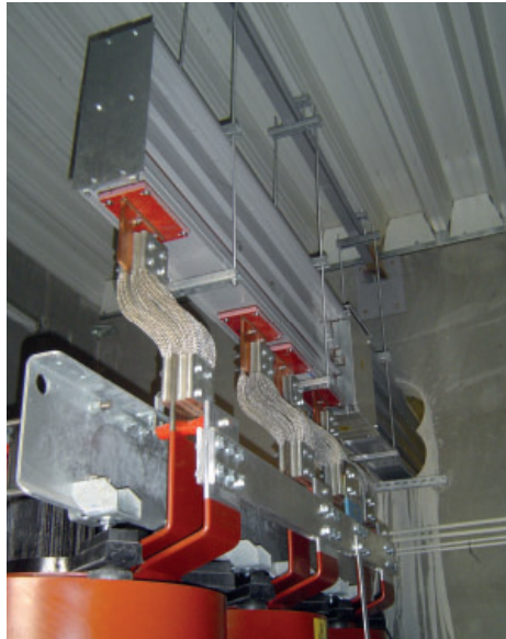
Type 1 busbar transformer connection and flexible braids.
