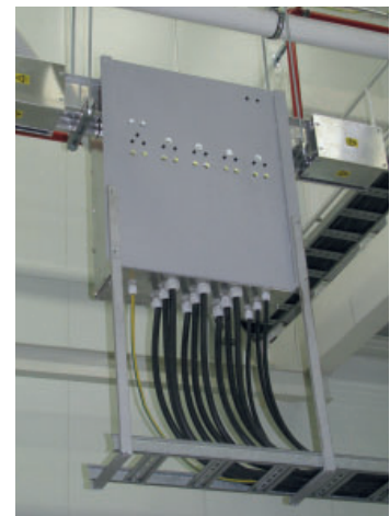
Centre feed made to accommodate multiple cables.
