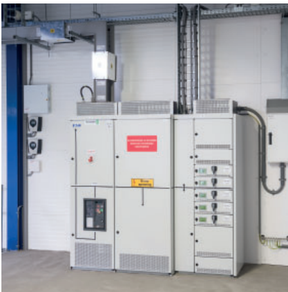
Eaton Capitole 20 switchboard.
