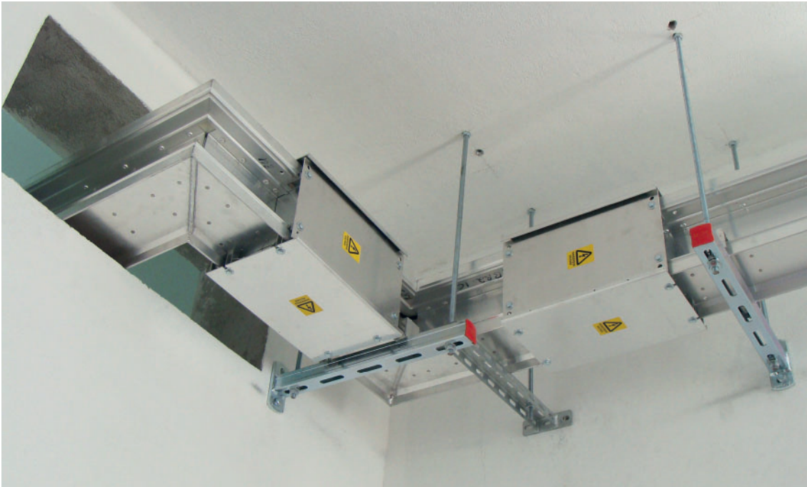
OTP Airport, Romania Power Xpert® XP.
