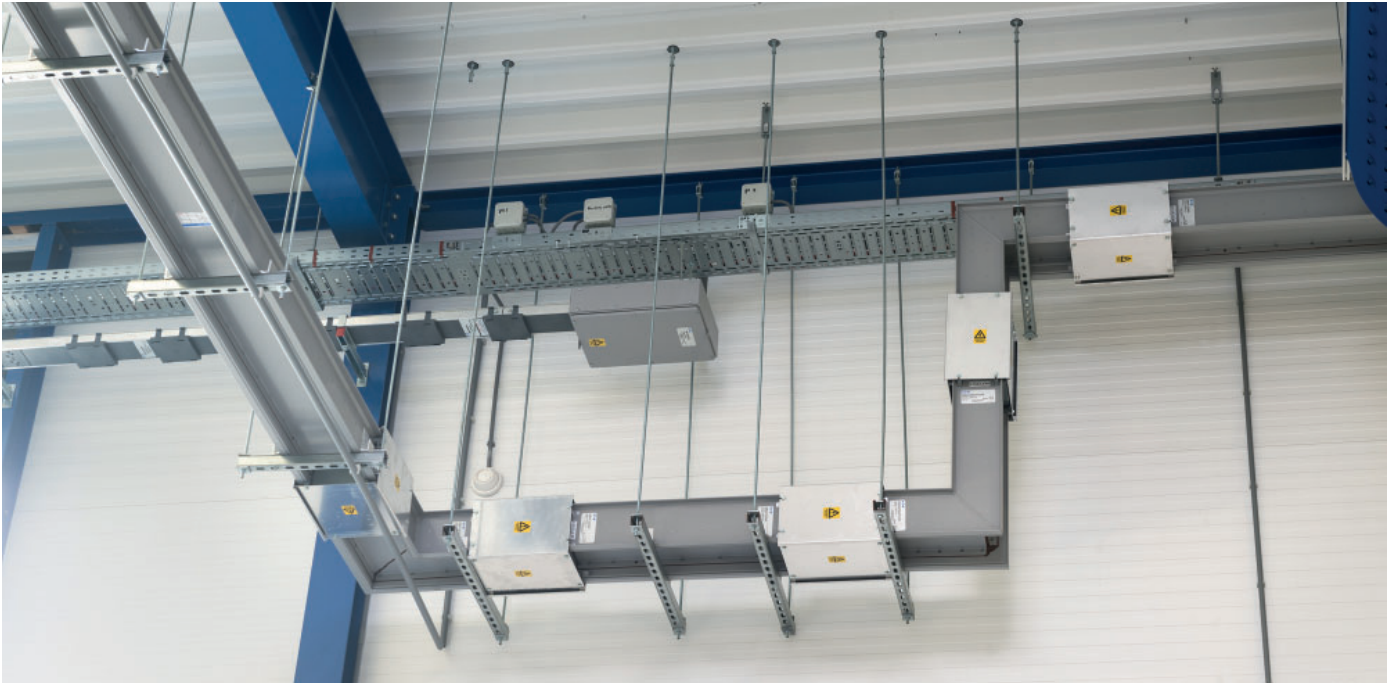
Galvano Techniek (industry), Hengelo (The Netherlands) Power Xpert® MP (Cu) at 160 A and Power Xpert XP (Alu) at 2000 A.
