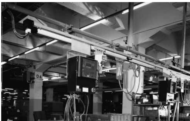
KTW-System in production line
