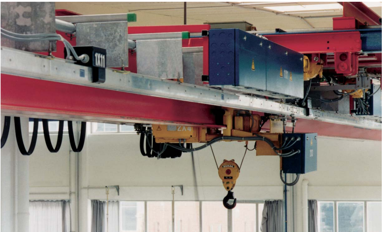
Aluminium enclosed conductor system LSVG on crane bridge.
